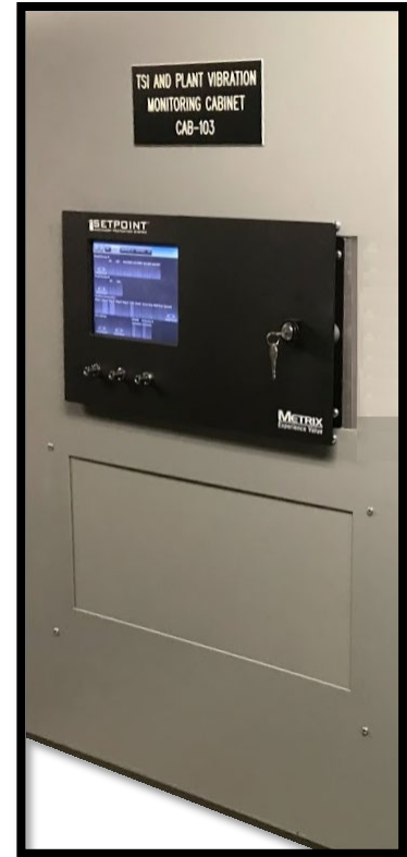
Figure 18: VC-8000 replaces a 3300 rack (same cut out).
